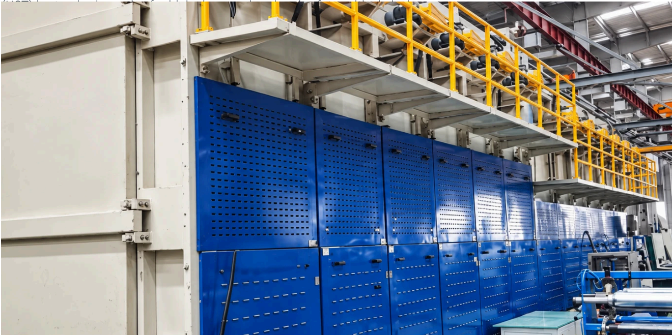
HEAT SOAK FURNACE
